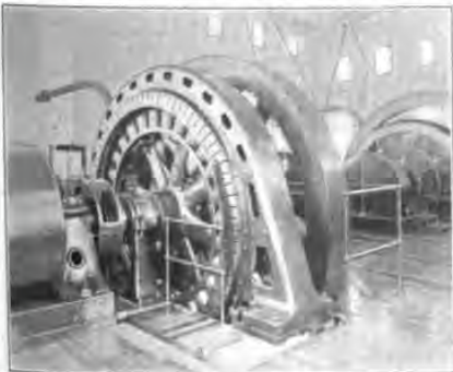
300 KW THREE-PHASE ALTERNATOR
